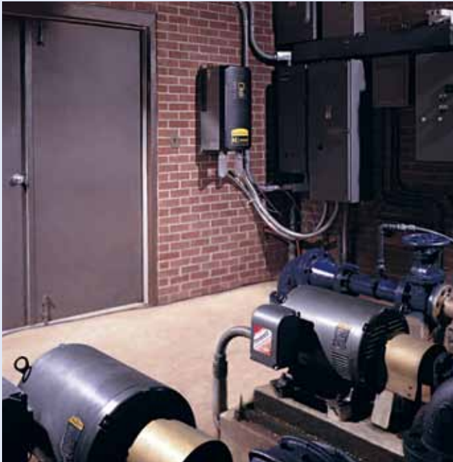
Baldor drives provide the additional benefit of preventing single phasing of the motors during power brownouts, saving the town from costly motor repairs or replacements.
